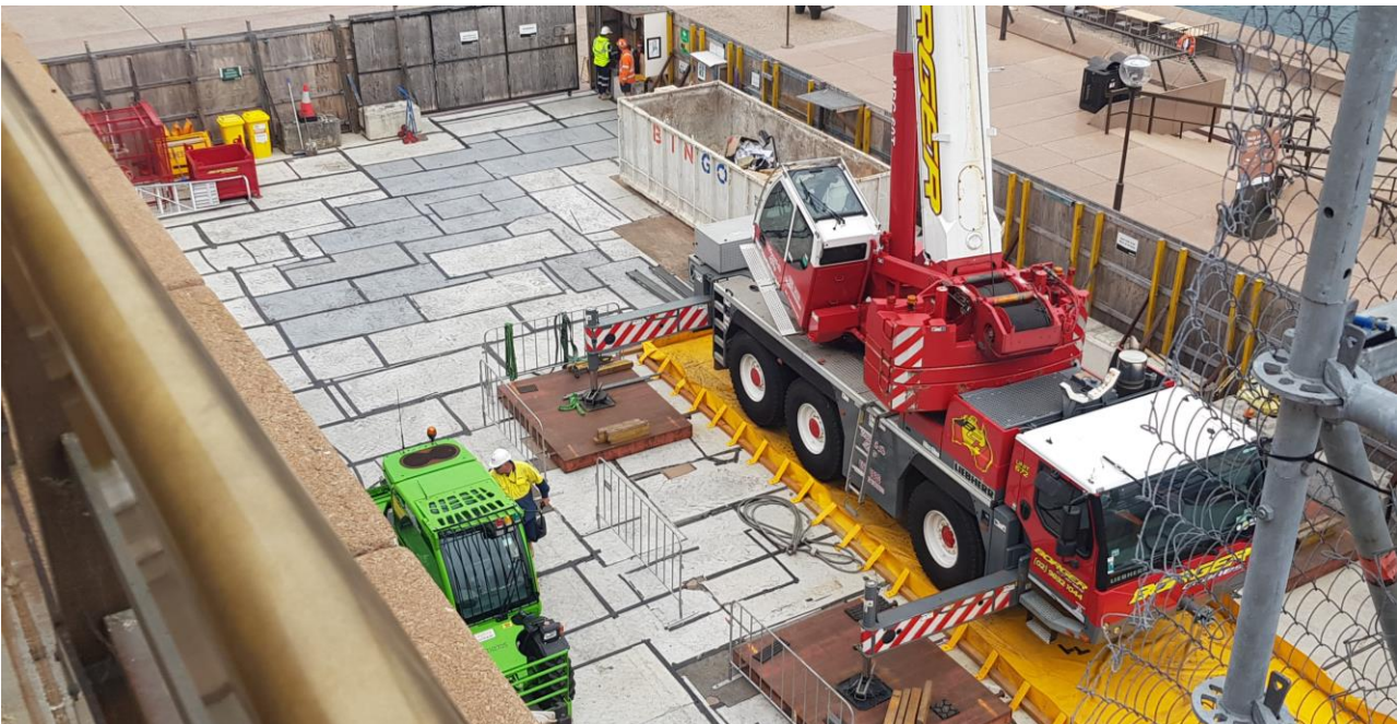
Photo 6: Overview of crane and telehandler work yard, with spill kits at entrance and bund under crane.
