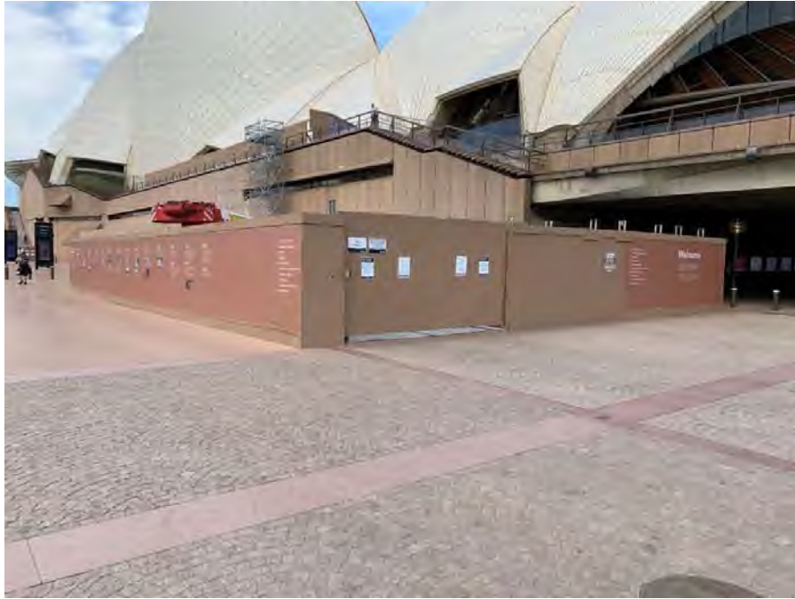
Construction hoarding around crane compound – heritage interpretation material along hoarding on Western Broadwalk
