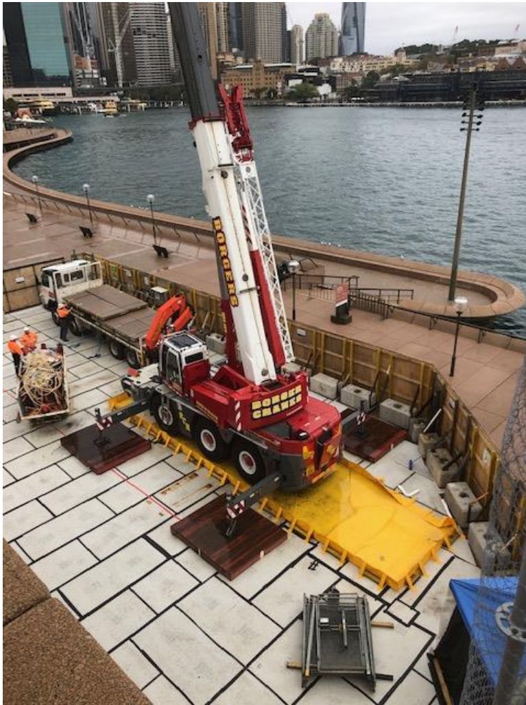
Photo 11: Crane parked within a bund to contain leaks (bund wall was mended during the audit)
