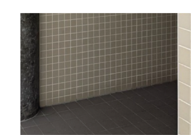
Ref Image - Site conditions 100 x 100 floor and wall tiling to match adjacent Male WC, as fitted beyond the entry Vestibule in 2021
